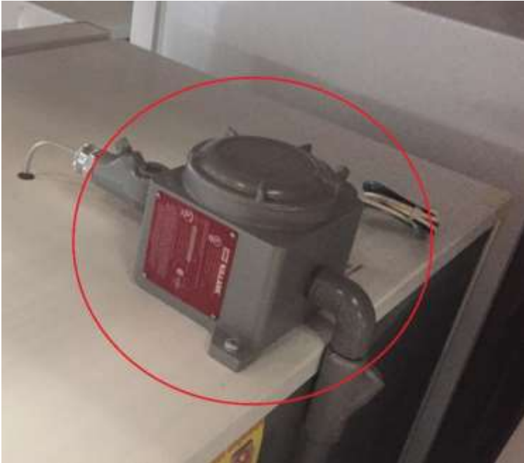
Mechanical Temperature Controller – located in the rear top location of refrigerator or freezer, inside of the metal enclosure.
